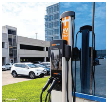
ChargePoint Level 2 EV charger at commercial building
